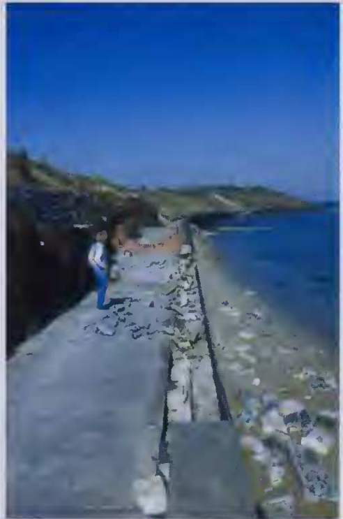
Fig. 7. Damage to sea wall by a previous storm, 30 April 1986.
